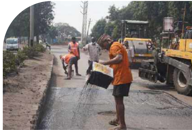
Repaired more than 18 km of village roads as well as fishermen approach roads in 4 sites - Mundra, Gangavaram, Jaisalmer and Raipur
