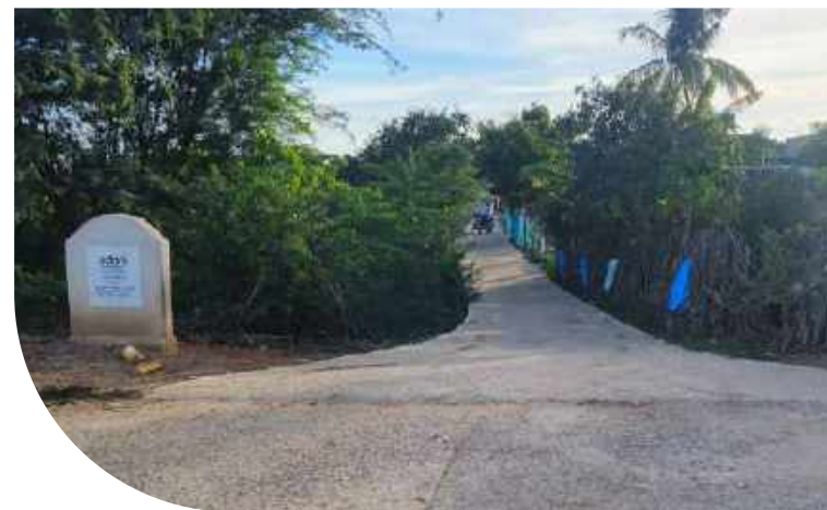
Constructed 20 CC roads of total 3,890 m of length in 6 sites - Mundra, Tirora, Kawai, Raigarh (Tamnar), Dhamra and Udupi
