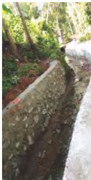
Renovation of Marian Nagar Drain, Vizhinjam (before)
