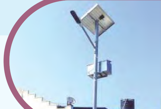
Solar Lights, Luvara
